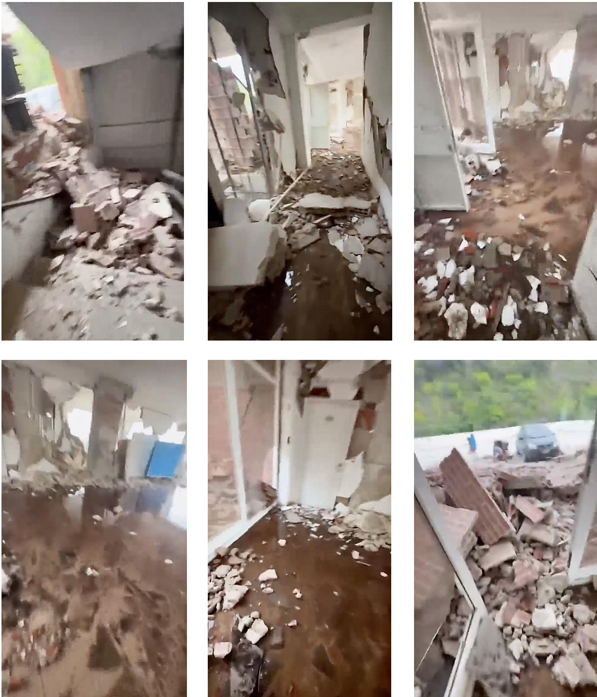
Figure A-5: Representative visual observations from the ground level. The observed conditions document the most severe damage encountered during the survey, characterized by extensive failure of unreinforced masonry infill walls consistent with apparent soft-story response mechanisms, while visible
