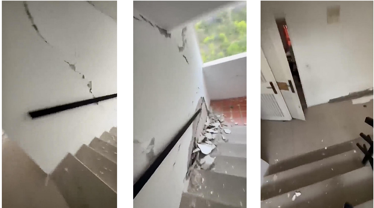
Figure 2: Intermediate story level demonstrating progressive in-plane shear cracking, minor plaster spalling, and initial debris accumulation on stair treads.
