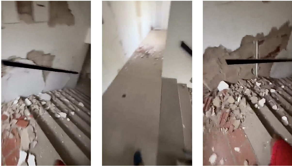
Figure A-3: Representative visual observations from the intermediate stories. The observed conditions indicate a progressive increase in damage severity compared to the upper stories, generally consistent with damage characteristics commonly associated with the Life Safety (LS) performance level defined in ASCE/SEI 41-17: (a) diagonal cracking and plaster spalling at stairwell landing walls, exposing the underlying masonry infill; (b) close-up view of extensive diagonal shear cracking in the masonry infill wall; (c) significant accumulation of masonry debris on stair treads and the landing; (d) view from the intermediate landing showing progressive cracking of the stairwell enclosure walls; (e) minor racking distortion visible at the corners of the door frame; (f) overall view of the stairwell illustrating the downward progression of damage; (g) increased accumulation of masonry debris on the stair treads; (h) corridor with accumulation of masonry debris; and (i) significant plaster spalling exposing the underlying masonry infill, accompanied by substantial accumulation of debris on the stairway.
