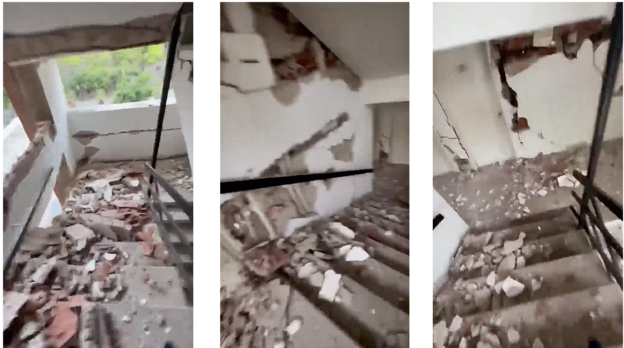
Figure 3: Lower story levels showing severe out-of-plane infill panel distress, large-scale plaster loss, and extensive debris accumulation on landing slabs.
