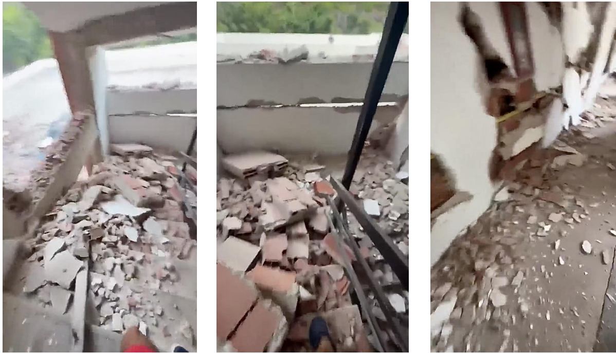
Figure A-4: Representative visual observations from the lower stories. The observed conditions demonstrate a pronounced escalation in damage severity compared to intermediate stories, generally consistent with severe nonstructural and infill damage approaching conditions associated with the Collapse Prevention (CP) performance level defined in ASCE/SEI 41-17: (a) Extensive collapse and loss of continuity of unreinforced masonry (URM) infill walls within the stairwell enclosure, with large portions of wall panels no longer intact; (b) and (c) wide vertical separation cracks within the corridor masonry infill walls, likely associated with seismic-induced incompatibility between the lateral deformation demands of the structural frame and the brittle response of the URM infill panels. Progressive frame–infill separation, combined with out-of-plane instability and localized dislodgement of masonry units, resulted in significant degradation of infill wall integrity, accompanied by cracking around door openings and separation between infill walls and surrounding frame elements; (d) extensive failure of stairwell enclosure walls with progressive loss of wall continuity across multiple stories, exposing exterior openings and adjacent building spaces; (e) widespread cracking, spalling, and partial detachment of masonry infill and finish materials at the lower levels; (f) similar conditions to those observed in (a) and (b), including severe deterioration and loss of continuity of URM infill walls; (g) complete failure of portions of the stairwell enclosure walls, resulting in significant loss of enclosure integrity; (h) substantial accumulation of masonry debris obstructing stair treads and landing slabs, limiting accessibility and indicating severe localized infill failure; and (i) conditions similar to those described in (a), showing extensive collapse and loss of continuity of URM infill wall panels.
