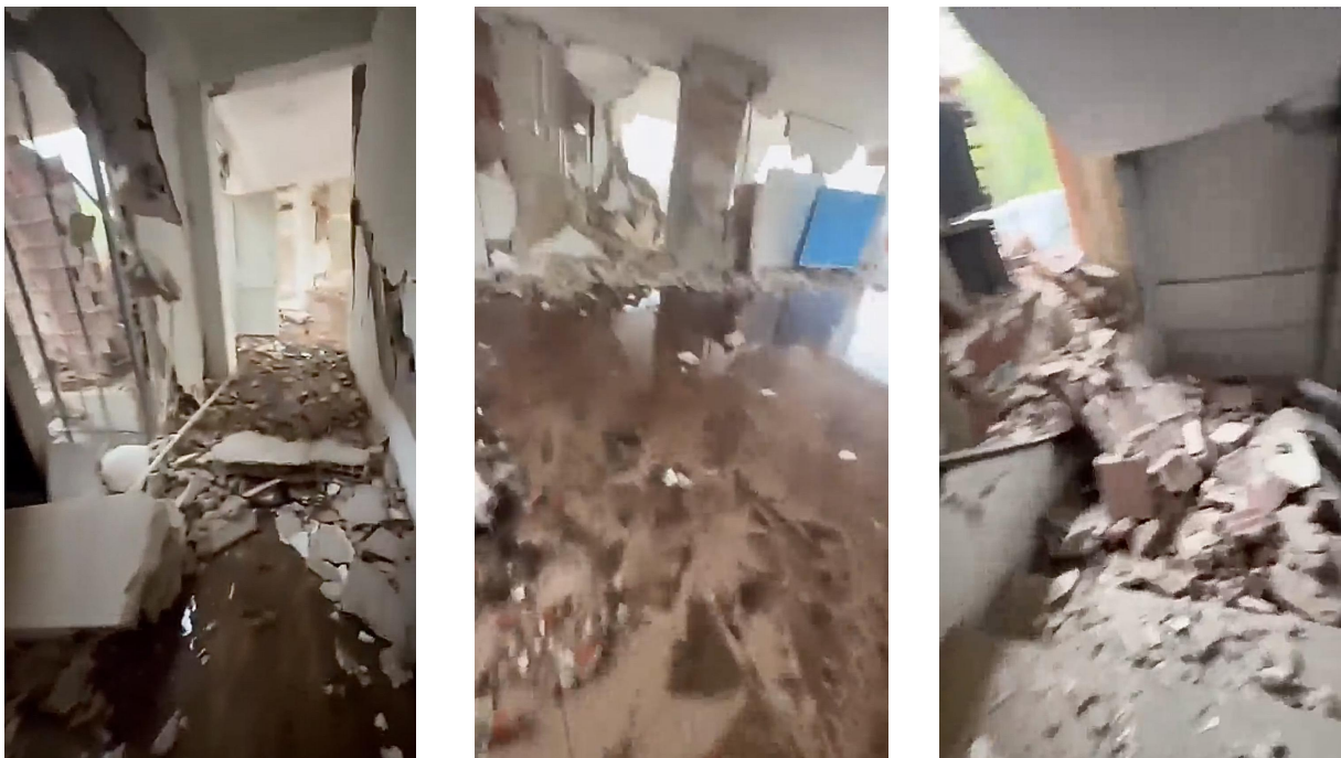
Figure 4: Ground-floor level and basement stair entry showing near-total masonry infill failure, heavy structural debris obstruction, and standing water from damaged MEP utilities.
